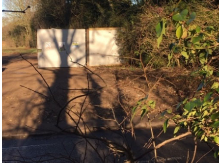
1 st November 2019, Hazel removal evident, with compaction and hard surfacing, tree root damage (and no tree protection) at construction access
